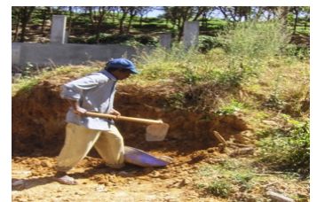
A male resident working at the construction site of our Biogas plant
